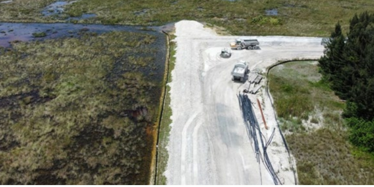
▲ The new seepage wall will reduce flooding in this community while allowing the remainder of the water to continue flowing through the Everglades. Photo: SFWMD
