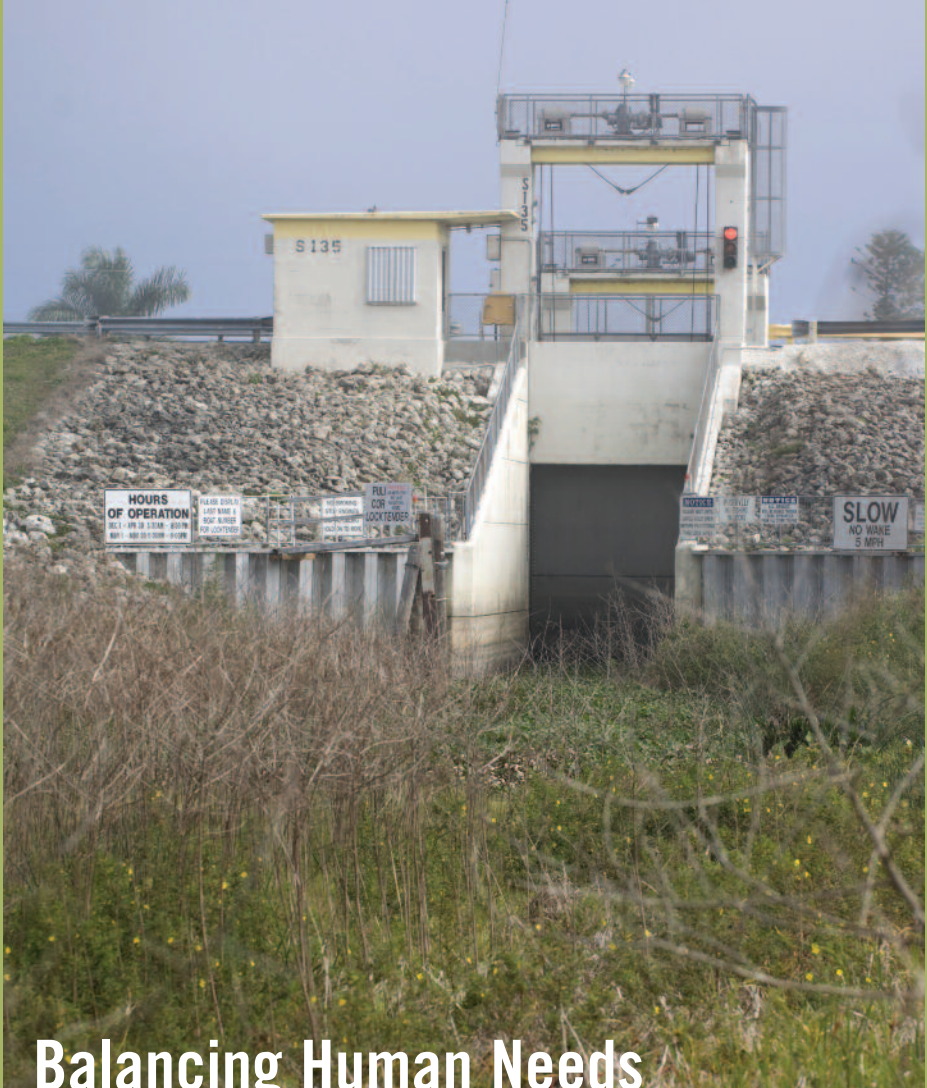
This grass-filled lock on the east side of Lake Okeechobee would, under normal conditions, be completely surrounded by water. Photo courtesy of South Florida Water Management District.
