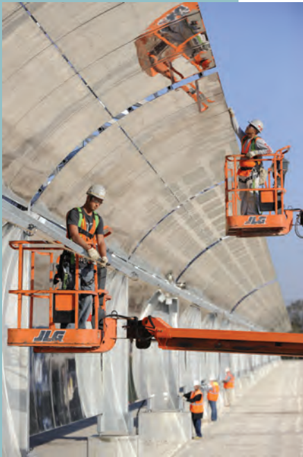
Workers install one of the 190,000 mirrors at Florida Power & Light Company's Martin Next Generation Solar Energy Center in Indiantown, Fla. The plant which opened in March created 1,000 direct jobs during construction.
